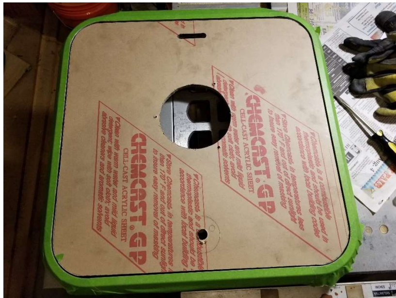
The new lens is in place and the first pass of Dowsil 795 is in the groove.
