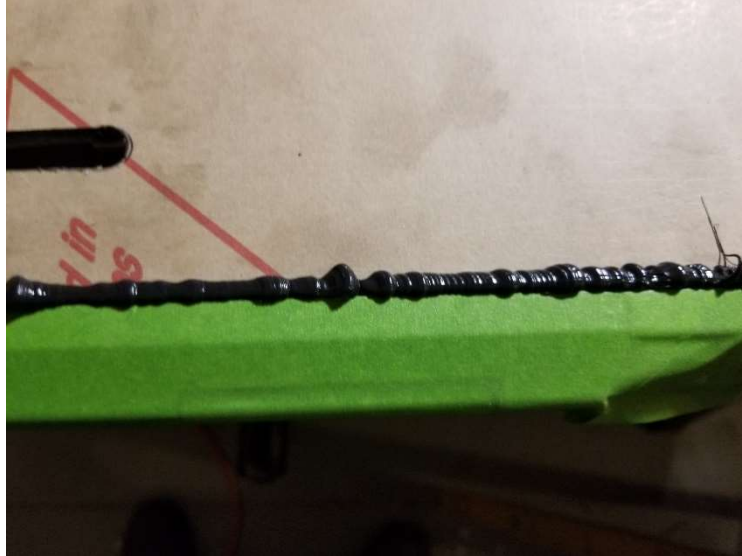
Close-up of the first bead of sealant before running my finger around the joint to smooth it.
